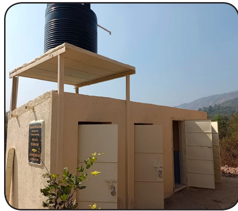
Renovation of Classrooms and Toilet, Raigad Zilla Parishad School, Morbe, Karanbele, Taluka Panvel
